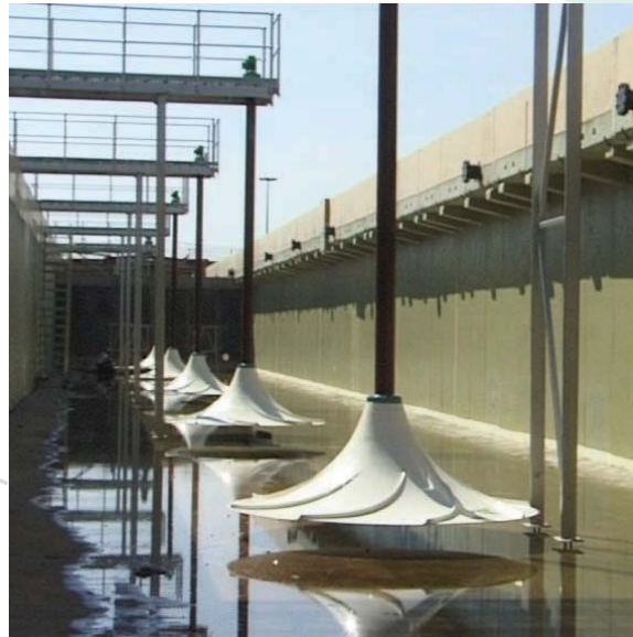
6 out of 116 HYPERCLASSIC® -Mixers in a wwtp in Berlin, Germany
