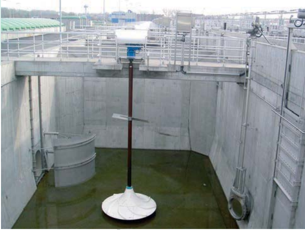
1 out of 32 HYPERCLASSIC®-Mixers in a large wwtp in Vienna, Austria
